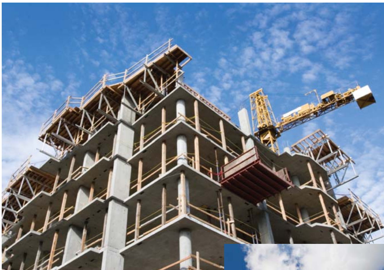
Construction Elevator Emergency Stops
